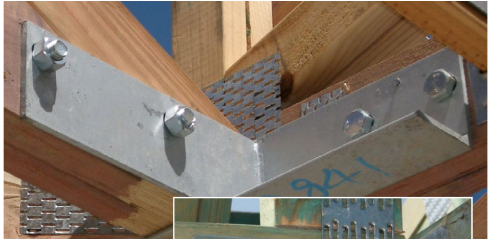
■ Photo 1 - Undersized bolt fixing
