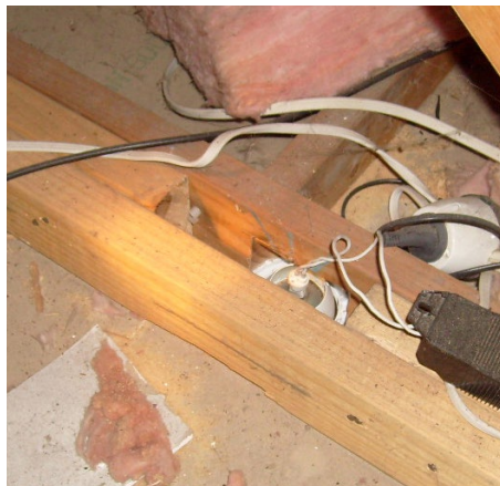
■ Photo 2: Could the down light not have been repositioned?
