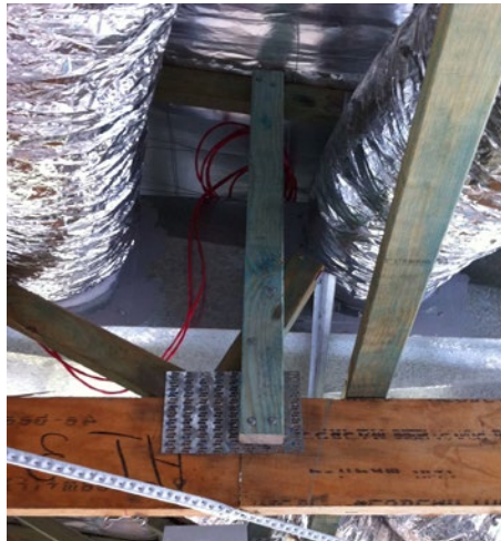
■ Photo 1: Could the ducting not have been moved over a little?
