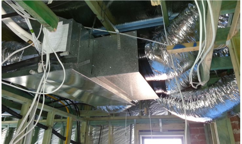
■ A poorly retro-fitted air conditioning unit.
