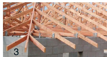
■ A worker risks falling off the roof when hip creepers are not supported by a structural fascia.
