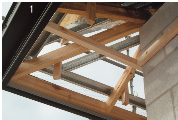
■ A structural timber fascia has been properly installed behind the metal fascia at a hip corner.
