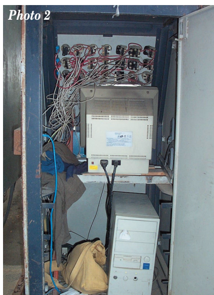
Photo 2 ■ Electrical cabinet or personal locker? Electrical cabinet access should be controlled.
