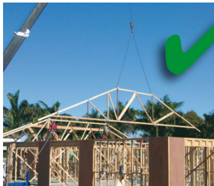
Right – This is a good example of how a truss should be lifted.
