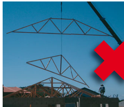
Wrong – Trusses should not be lifted from a single point, and especially not from the apex nor from mid-panel between joints.
