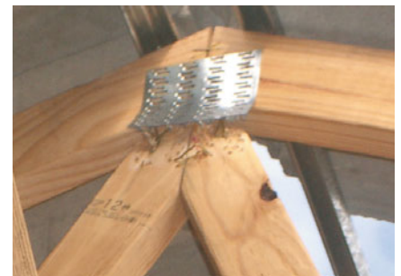
This apex plate of a girder truss failed under load because it was weakened by being lifted from the apex.
