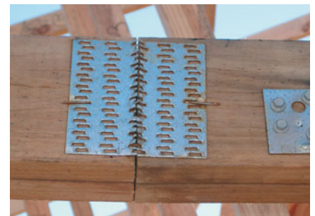
This plate was torn because the heavy double truss was lifted flat on its side from the middle causing severe flexing and stress.
