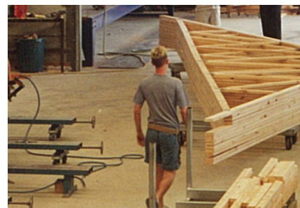
■ Many plants lack the space for truss outfeed rollers for safe truss removal.
