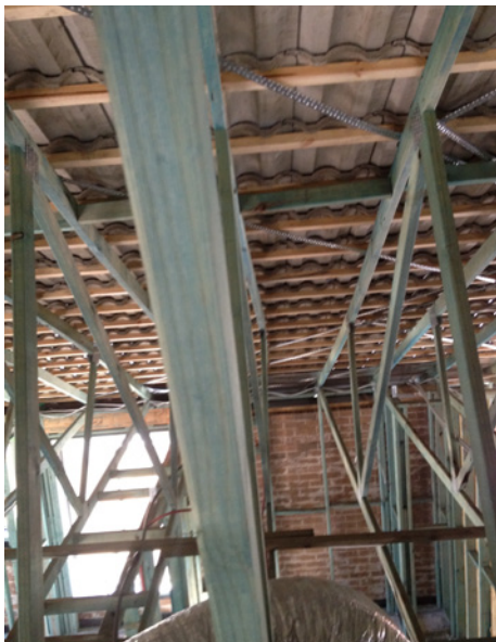
Photo 1: Top chord outside the required limits of straightness.
