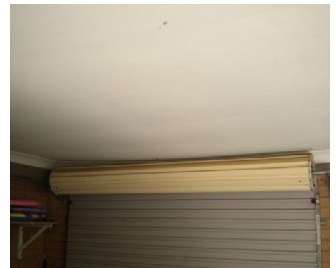
■ Detached ceiling resting on roller door.
