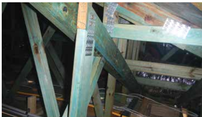
Photo 1: Incomplete nailing along the supplementary top chord.
