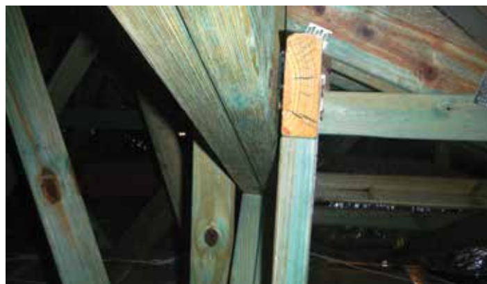
Photo 2: Screws not fully driven home.
