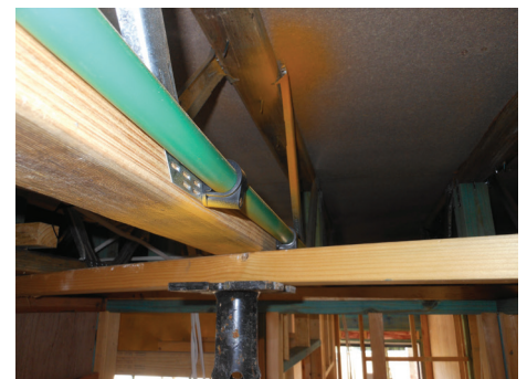
Image 4: Neither prop nor timber plank were securely fixed.
