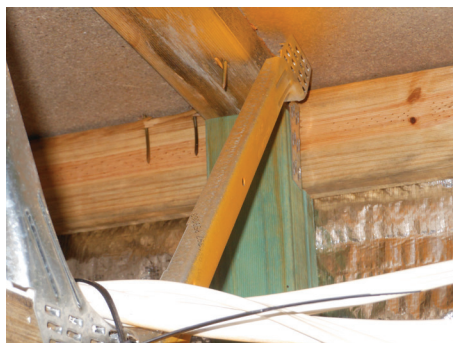
Image 3: Overloading caused the webs to dislodge.
