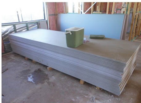
Image 1: Plasterboard stockpile overloading the floor.
