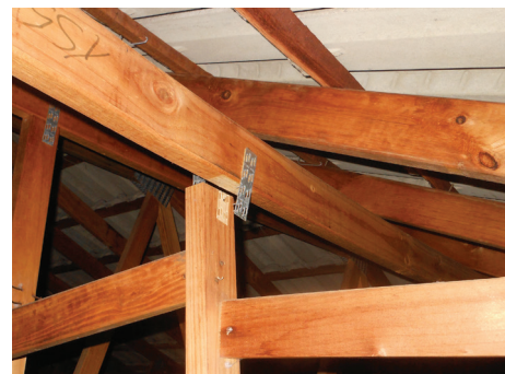
Dislodged plates from twisted trusses.
