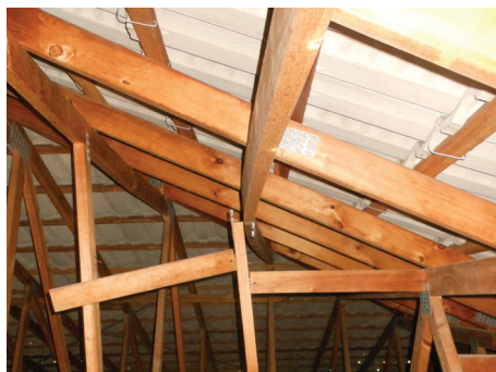
Badly bowed trusses from lack of fixing.
