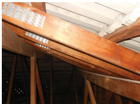
Absence of fixing between rafters and trusses.
