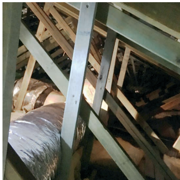
Above: a veritable forest of extra timbers added to trusses, which were in turn packed off an internal non-loadbearing wall. When checked, the bottom chords were found to have hogged upwards by up to 20mm!
