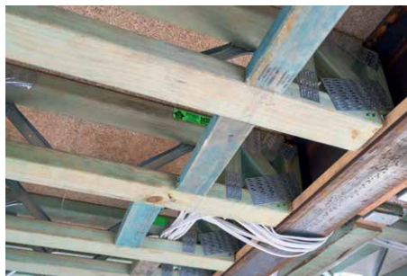
Figure 1: Tolerances allowing for some steel beam flexibility. Courtesy of Colli Timber & Hardware and Bellissimo Homes.
